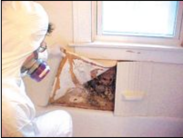
Photo provided by Sanit-Air in Troy Wearing protective clothing and a respirator, inspector Connie Morbach of Sanit-Air in Troy finds mold behind tiles in a bathroom.
